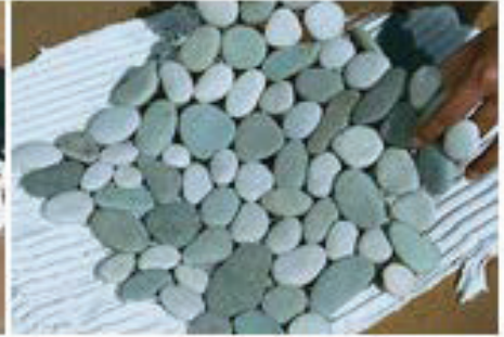
Place tiles on the thinset. Take extra care to get each tile close together using their interlocking shape.
