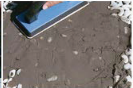
Apply a sanded grout on 2"x2" sections at a time until the entire installation is covered.
